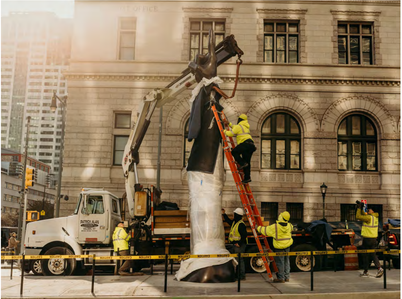
“Unity,” 22 feet tall, being installed near the intersection of Adams Steet and Tillary Street in Brooklyn. Kyle Johnson for The New York Times
